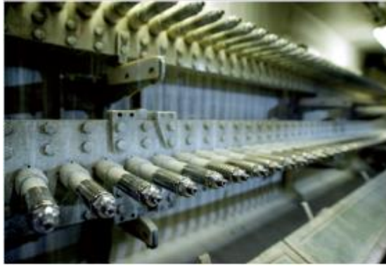
Figure 9– Spray nozzles in the coater
